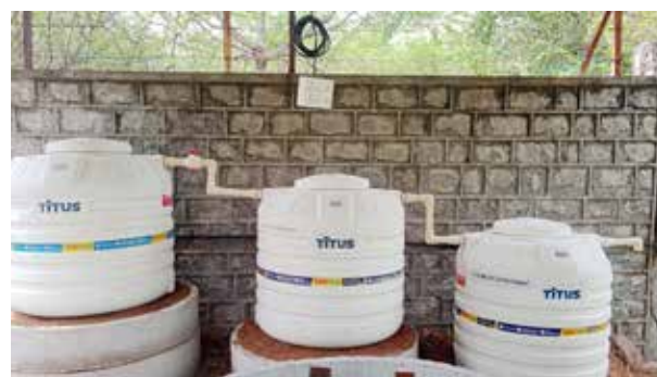
Portable wastewater treatment unit
